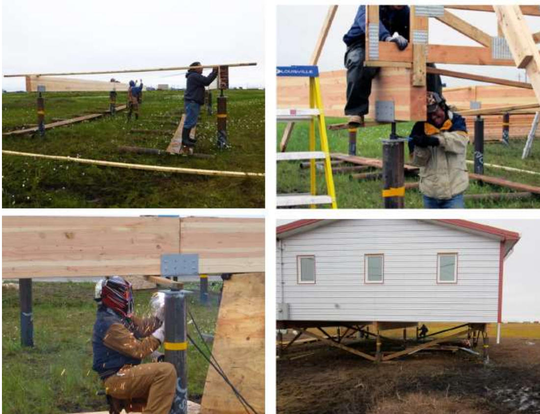
Figure 26. Example use of Saddle Bracket jacks over piles to adjust elevation due to soil settlement resulting from thawing effect in active layer and permafrost zone (CCHRC 2014)
