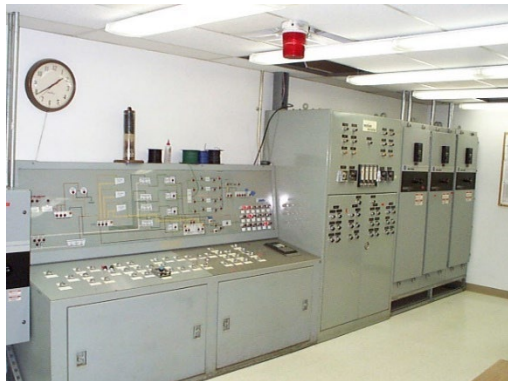
Girdwood Wastewater Treatment Plant
