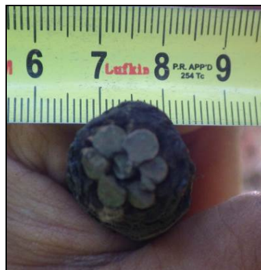
Figure 40. Detail of one end of the electrical cable recorded at Test Unit 57 (NLURA photograph).
