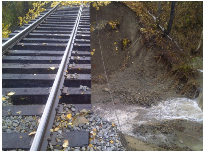
Major washout just south of Gold Creek.
